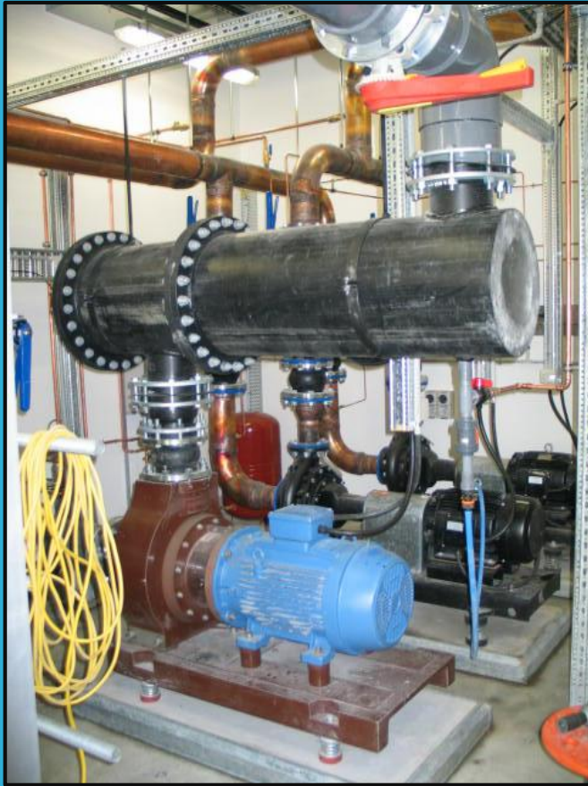
Seawater heat exchange filter and pump
