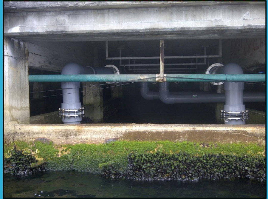
Seawater heat exchange piping below wharf
