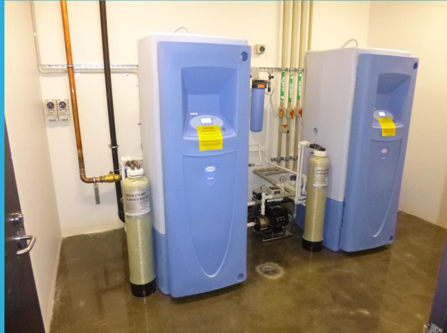
Reverse osmosis water plant
